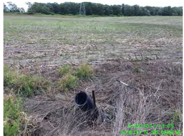
Photo #52 Main east-west tile inlet, east side of property near driveway, view southeast.
