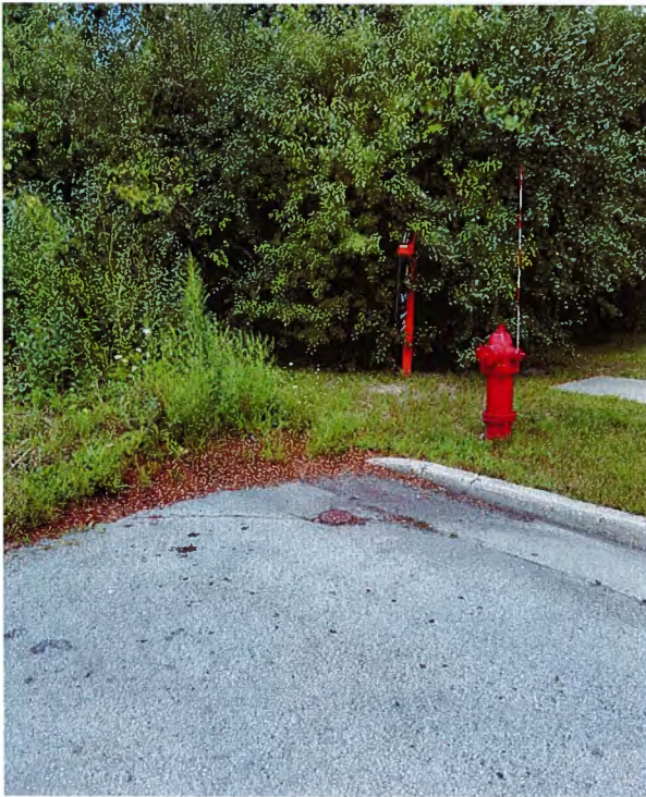
Figure 5. Proximity of fire hydrant to the dead-end located at the west end of W Lake Pointe Drive.
