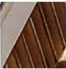
SOFFIT - PRE FINISHED ALUMINUM SOFFIT PANELS WITH CONTINUOUS VENTS (COLOR TO MATCH FASCIA)
