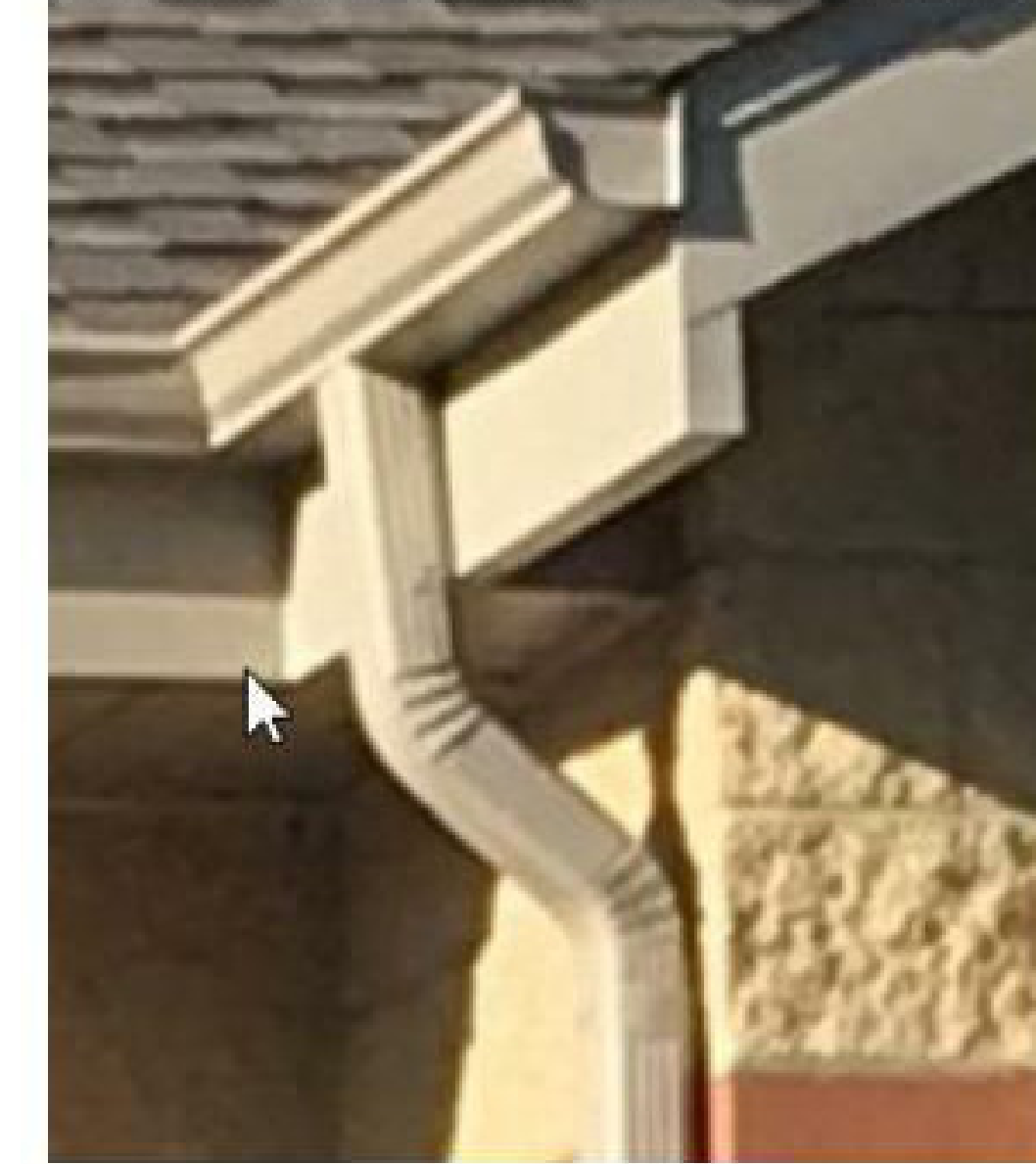
PREFINISHED METAL DOWNSPOUT AND GUTTER SYSTEM
