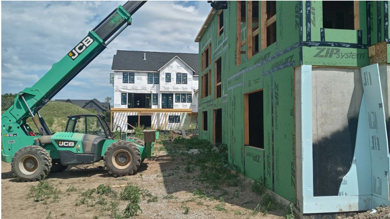
View of the rear yard where the subject deck is being proposed Photo by City Development staff
