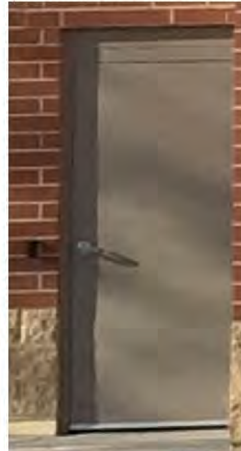
PAINTED HOLLOW METAL SERVICE DOOR AND FRAME (COLOR TO MATCH ADJACENT MASONRY).
